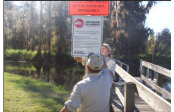
Bob Craft and Larry Irvin with Leisure Services Division installing sign at the Peace River Canoe launch in Bartow.
